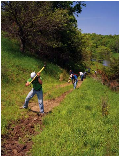
Building trail in the Whiterock Conservancy. Photo courtesy of Steve Milanowski / Whiterock Conservancy
